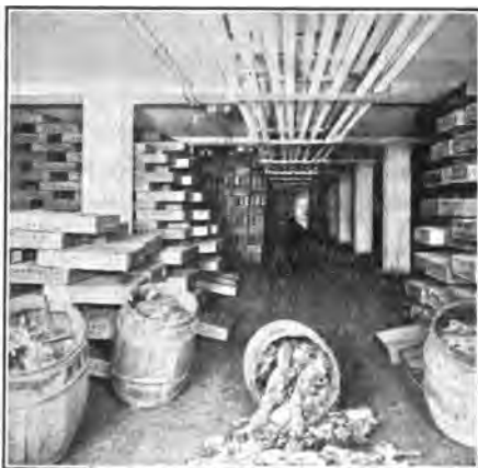
FIG. 47. — A cold storage room. Notice the frost-covered pipes overhead.
